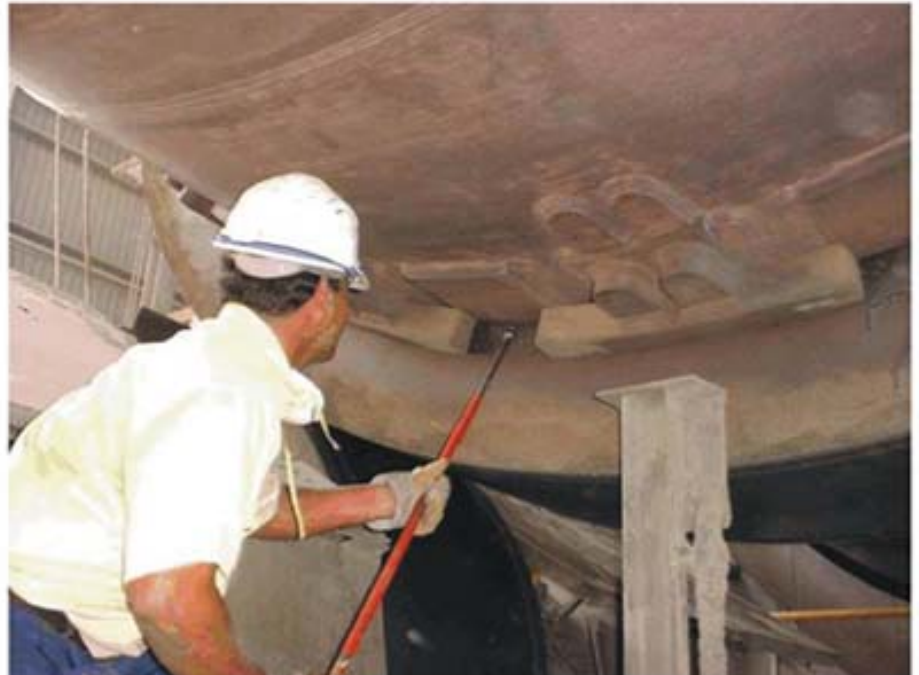
Application of BERULUB VPN 13 RINGLUB by a Knappsack Spray Unit at a Rotary Kiln in a Cement plant
